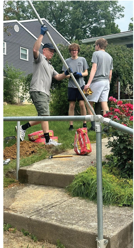
Retired Command Sgt. Maj. Mike Boyd, left, president of AUSA's Maj. Samuel Woodfill chapter in Cincinnati, helps install aluminum handrails at the home of local Army veteran Richard Walsh. (AUSA PHOTO)
